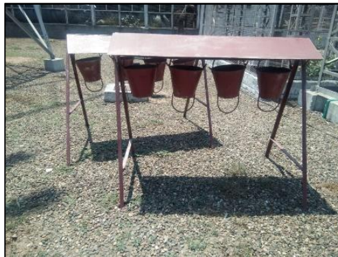
Photographs of the fire extinguisher provided within unit
