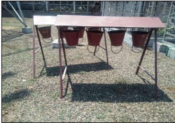
Photographs of the fire extinguisher provided within unit
